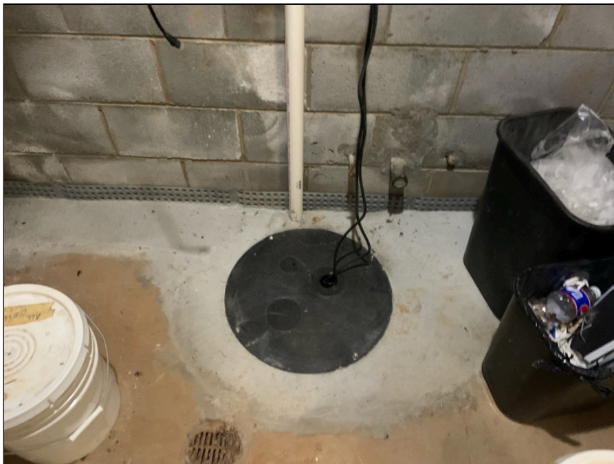
8 - Sump pump located in the basement of 458 N Madison Road
