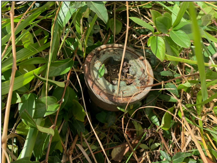
16 - Fill port located along the southern exterior of 454 N Madison Road
