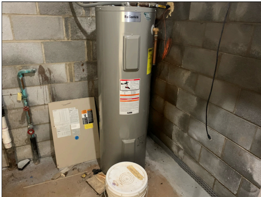
4 - Hot water heater closet in the basement of 458 N Madison Road
