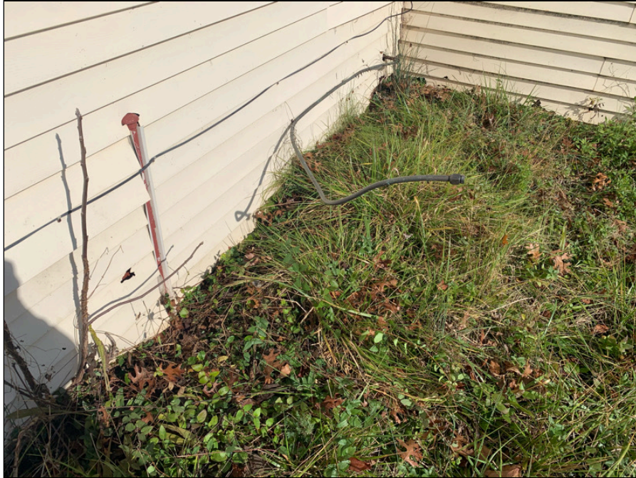
15 - Vent pipe and piping located along the southern exterior side of 454 N Madison Road
